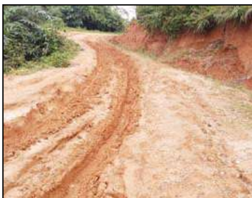
Earthen Road start at 15.8Km, proposed for JGT application for strengthening of pavement
