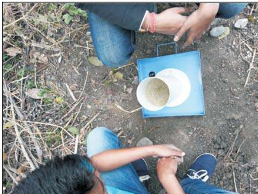
Measurement of Field Dry Density of Soil by Sand Replacement Method at Road Site in Manipur
