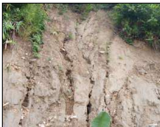
A View of an Eroded Spot of Uphill Slope
