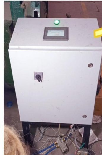
Control panel with HMI Screen
